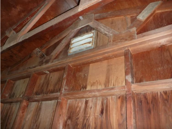
Photograph 8: Electrical Vacuum Building
