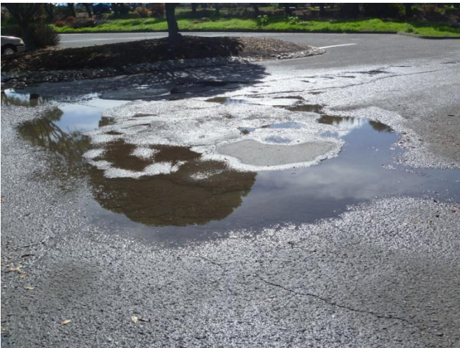
Photograph 9: Potholes & Alligator Cracking
